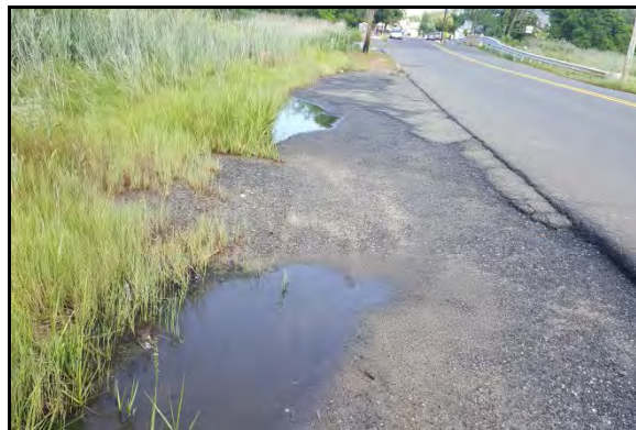
Figure 172: Flooding along Chingarora Creek on First Street between bridge & Walnut Street on a “dry” day (August 18, 2016)
