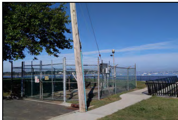
Figure 159: Pump station at Cedar Street bulkhead (September 23, 2016)
