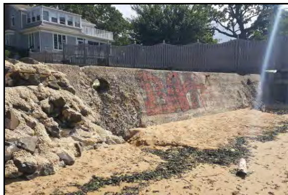
Figure 167: Concrete bulkhead and outfall pipe at Walnut Street at Keyport Harbor beachfront (August 18, 2016)
