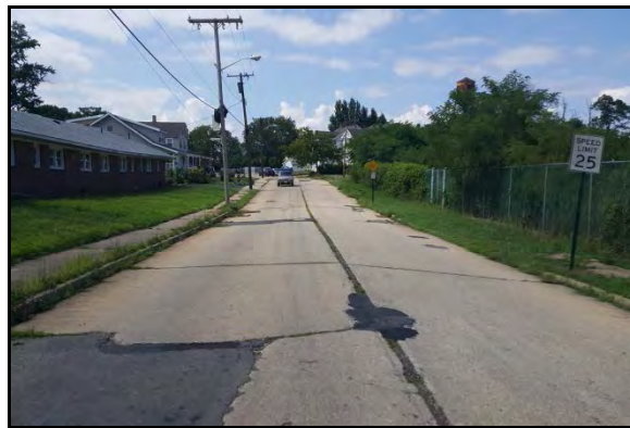
Figure 170: Conditions on Walnut Street (August 18, 2016)
