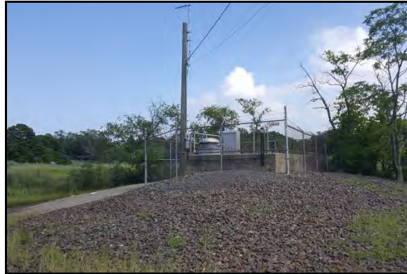
Figure 160: Pump station at First Street (August 18, 2016)
