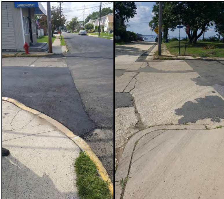
Figure 178: Ramps force pedestrians into the middle of oncoming traffic at Fulton & Second Street (left); No ramp is provided on some intersection corners, such as Locust Street at Walnut Street (right)
