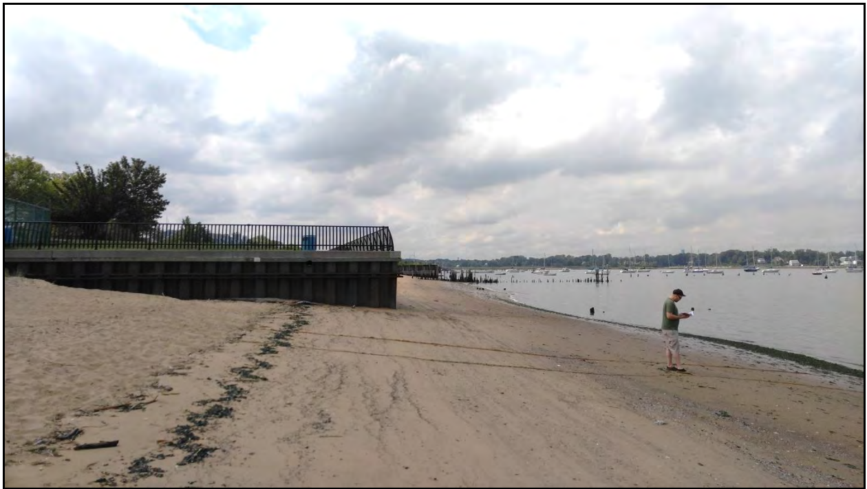
Figure 147: Hard structures along the bayfront, such as the bulkhead at Terry Park, are vulnerable to and often exacerbate erosion of surrounding sediment if significant wave action occurs (August 18, 2016)
