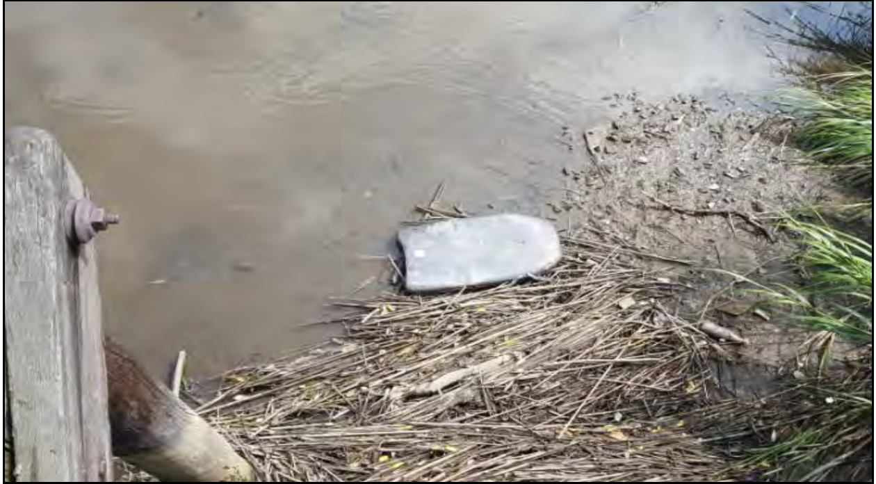
Figure 140: Example of accumulation of natural materials and pollution by bridge over Chingarora Creek (August 18, 2016)
