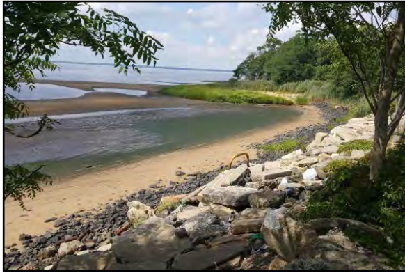
Figure 169: Riprap (stone and concrete pieces) along Aeromarine site waterfront on Raritan Bay (August 18, 2016)
