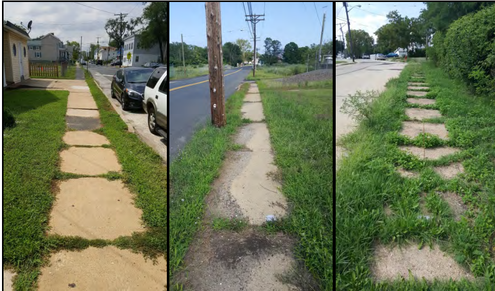
Figure 171: Examples of sidewalks in poor condition with overgrowth throughout the Walnut-Oak Neighborhood (August 18, 2016)
